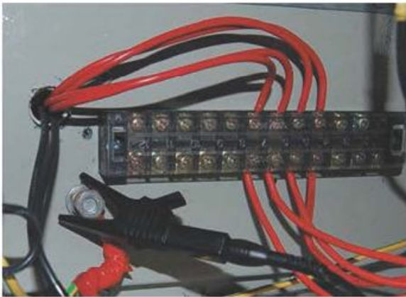
Application as connection to earth bolt in testing
